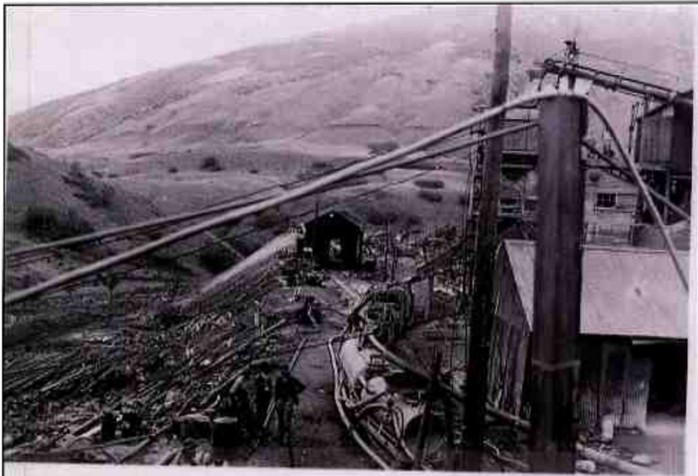
A-41-196 Concrete setup, Draper Portal. Batch plant, mixer gun, tanks, and shooting line. 10-24-41--Bur. of Reclamation photo., L. R. D.
