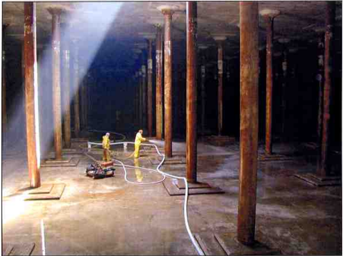
District employees cleaning the inside of Terminal Reservoir. The Reservoir must be completely drained in order to clean the inside.
