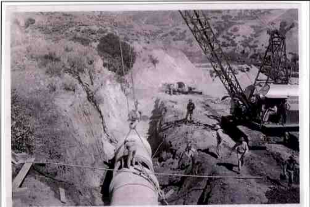
PR-712 Deer Creek and Salt Lake Aqueduct Divisions. Laying 69-inch diameter concrete pipe weighing 22 tons per 20-foot section. Laying up the line from the Utah Power & Light Company's flume at Station 491+ of the Salt Lake Aqueduct. 6-28-44--Bur. of Reclamation photo., L. R. Dunkley.
