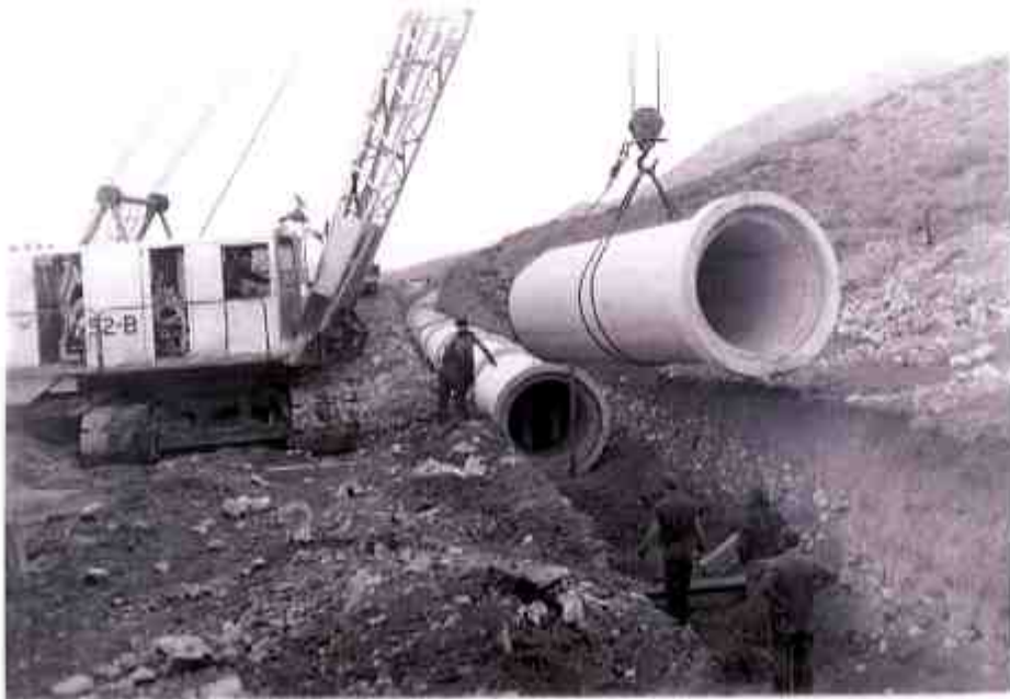
A-41-69 Lowering 69 inch diameter concrete pipe into place. 2-29-41--Bur. of Reclamation photo., L. R. D.
