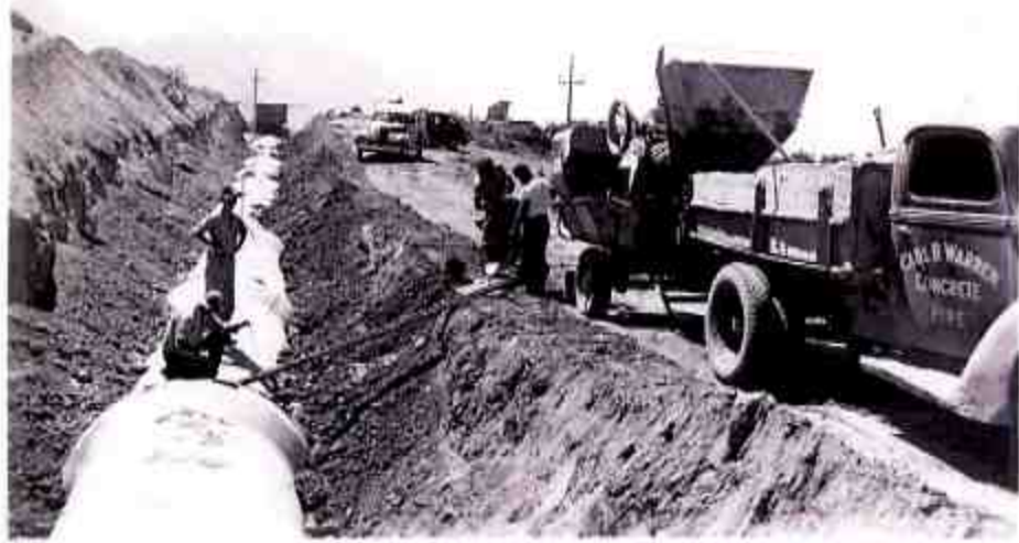
A-41-131 Grouting equipment outside jointing operations S.L.A. Upstream Station 575+50. 6-11-41--Bur. of Reclamation photo., L. H. D.
