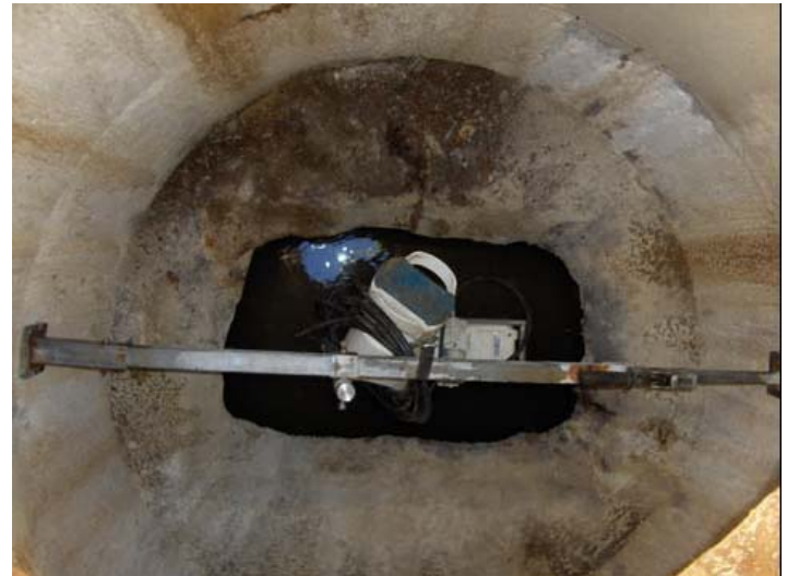
Pipe overflow Thanksgiving, 2005
