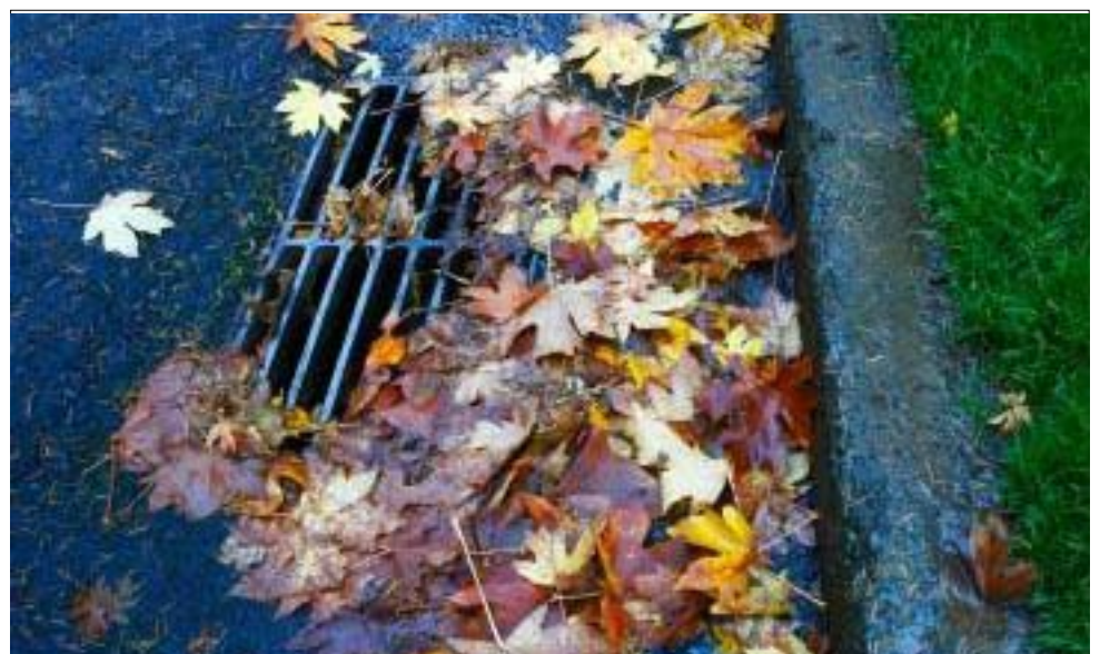
Look familiar? This is a common occurrence in fall. Leaves end up in the storm drains across the county and contribute to the low DO problems in the Jordan River
