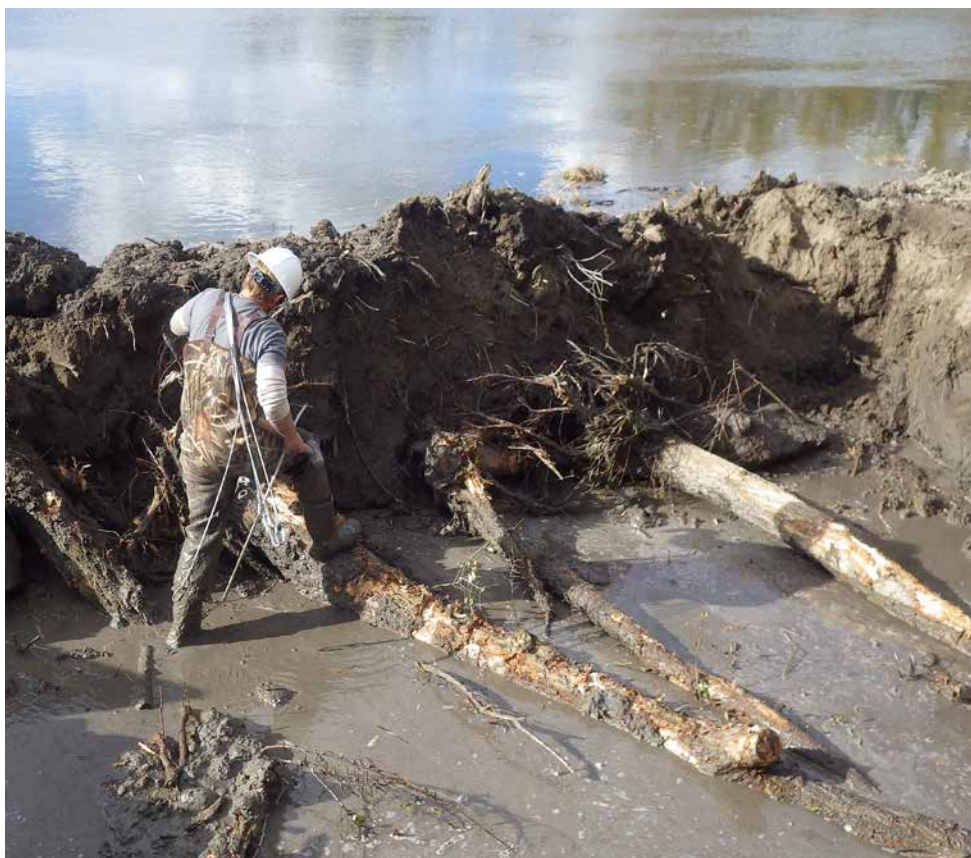
County Watershed crew member standing on the lower trunk of a toe-wood structure (closest to the root wad) to stabilize the trunk during installation.
